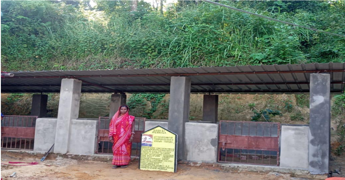
Photo: KHOWAI_TELIAMURA_UTTAR KRISHNAPUR _CONSTRUCTION OF PIG SHELTER _2020_ ABALA MALLIK. (Jobcard No:- TR-01-007-016-001/40. Aadhar No:- 2777-4354-5724.)
